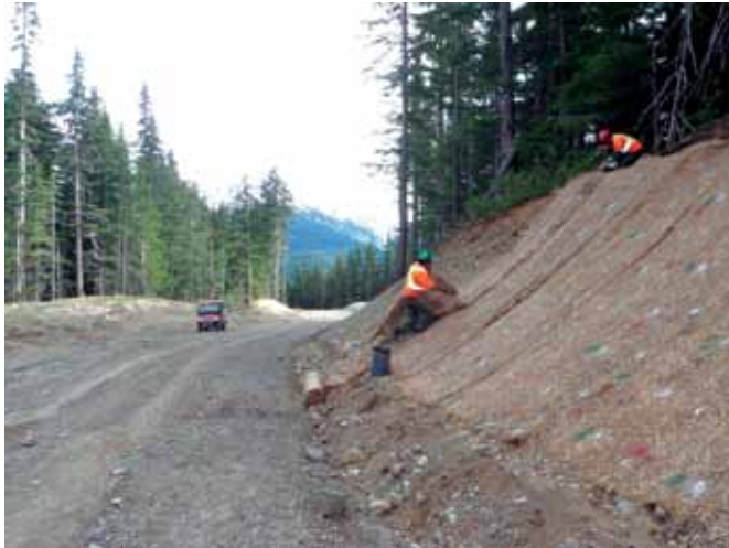
SLOPE STABILIZATION ALONG THE GALORE CREEK ACCESS ROAD INCLUDED INSTALLATION OF EROSION CONTROL BLANKETS
